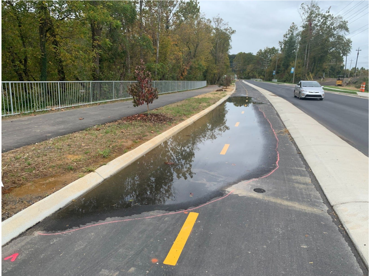
An example of pooling in the two way protected cycle track obstructing both lanes of travel outlined in chalk.
